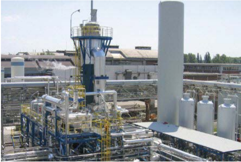
Figure 10: Haldor Topsoe green ammonia plant, being built in Saudi Arabia, capable of producing 650 tonnes a day.
