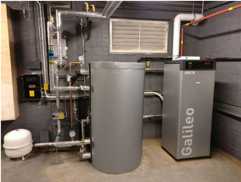
Figure 8: HEXIS Galileo 1000N 1 kWe CHP system installed at the University of St Andrews. The system utilises a solid oxide fuel cell stack
