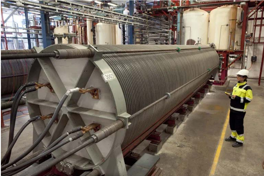
Figure 7: Alkaline electrolyser stack at Akzo Nobel 10
